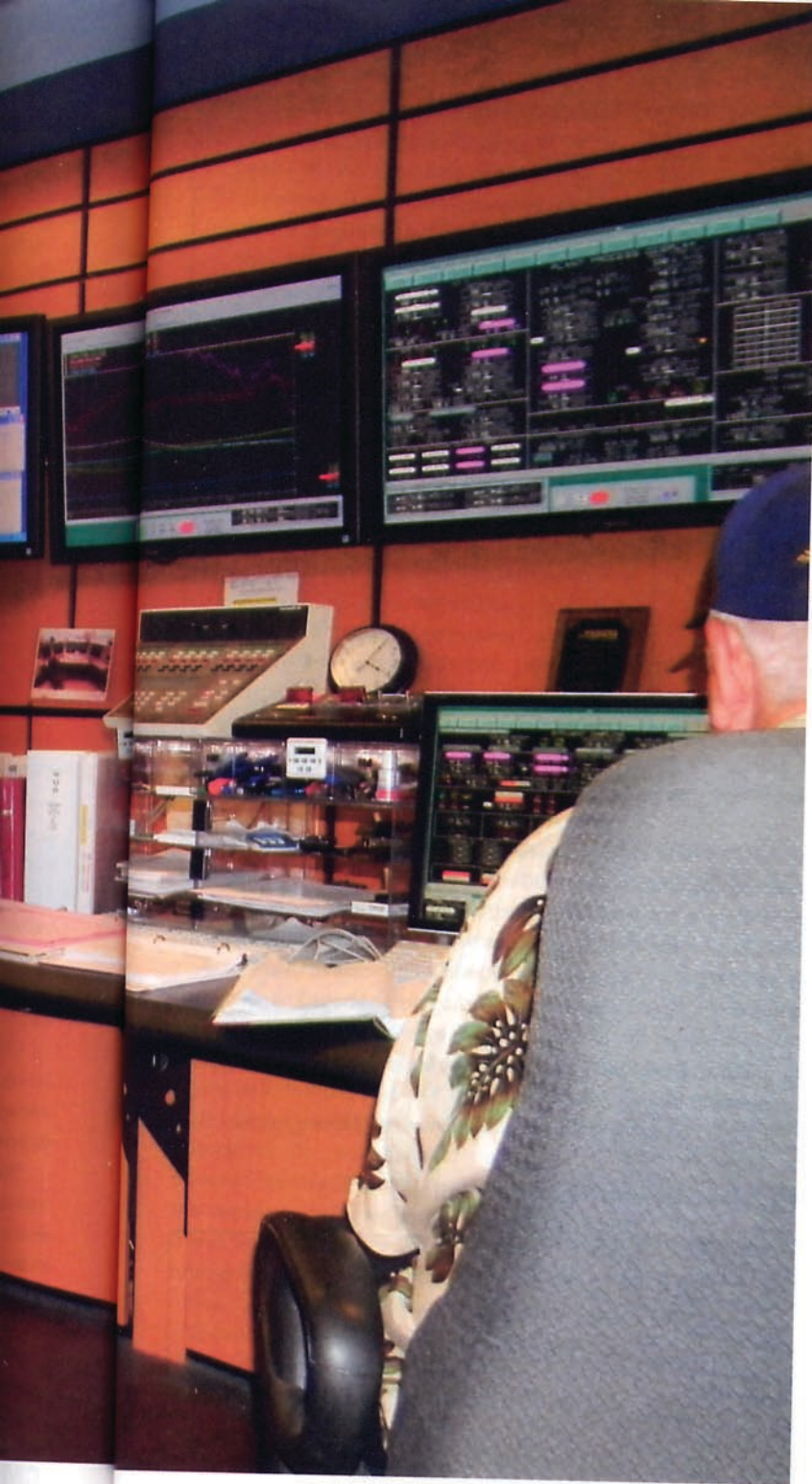
◀ Operations staff monitor processes from the Sacramento (Calif.) Regional Wastewater Treatment Plant control center. Joshua Nurmi
